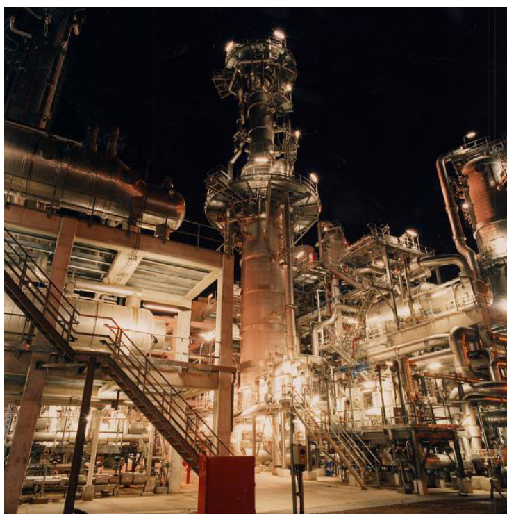
Figure 4. An Air Products MCHE in service showing the completed platform and piping structures (courtesy of Oman LNG).
